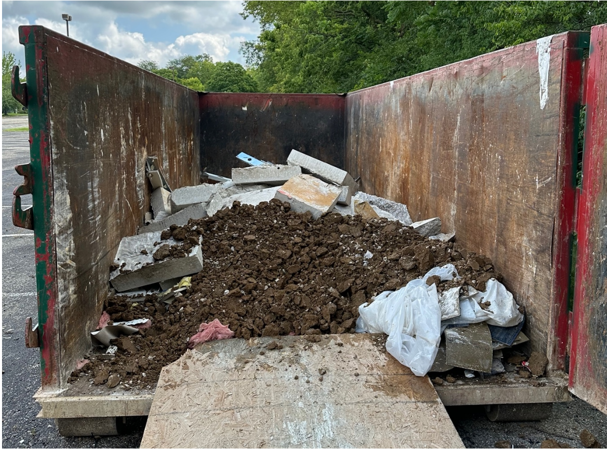
Concrete from KC bathroom drain
