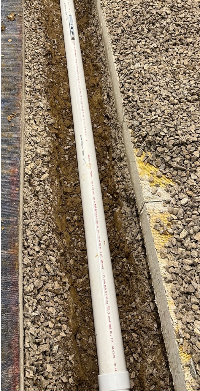
KC floor drain:
